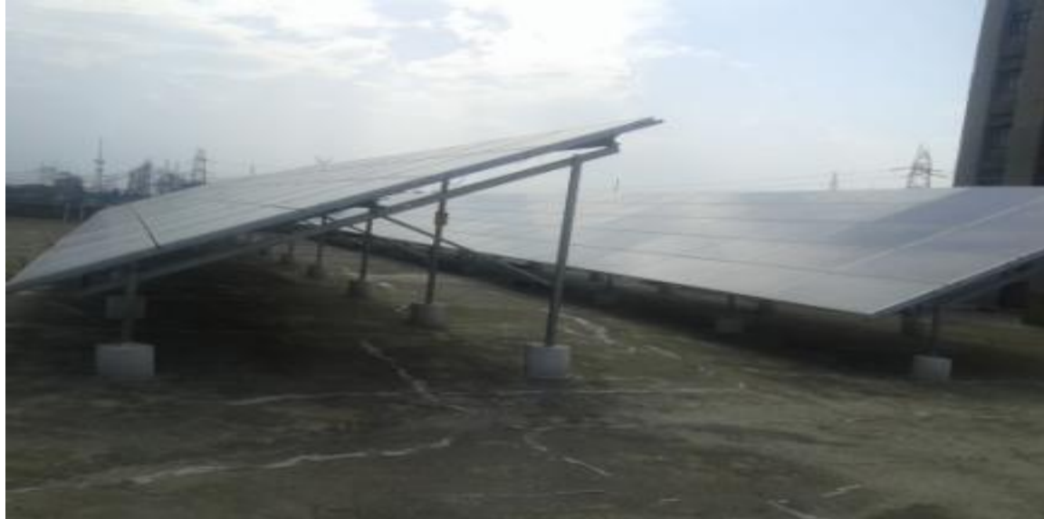
50 KW SOLAR PLANT AT NTPC SIPAT SIMULATOR BUILDING
