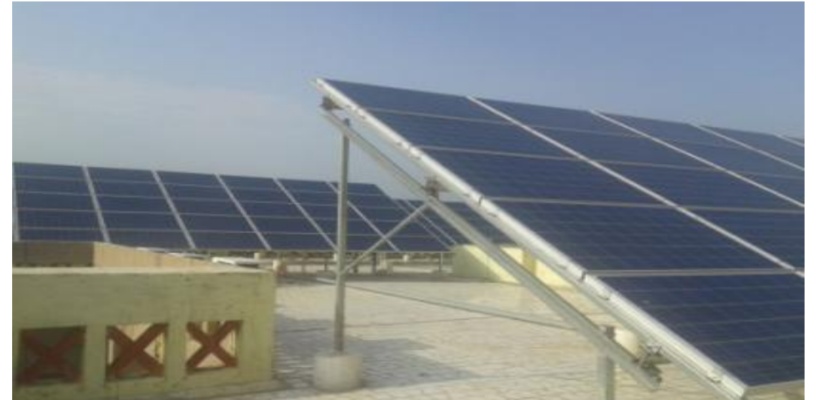
100 KW SOLAR PLANT AT SIPAT EMPLOYEE DEVELOPMENT CENTER & HOSPITAL ROOF
